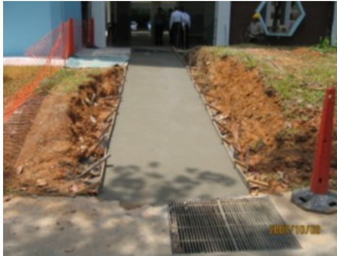
Figure 26: Photo of non-suspended pavement slab taken at Simei HDB Interim upgrading project
